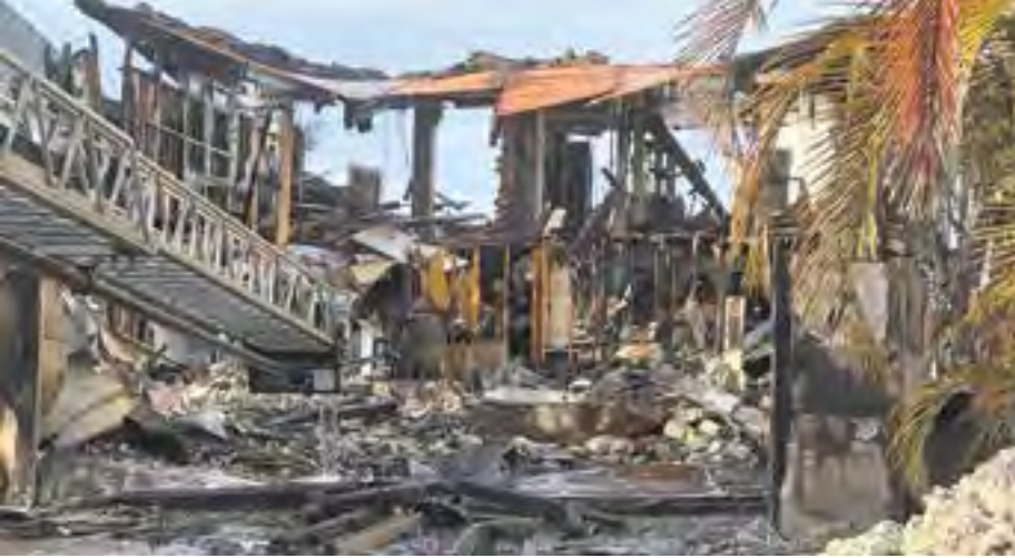
A beachfront home is left destroyed by a fire during a storm.
